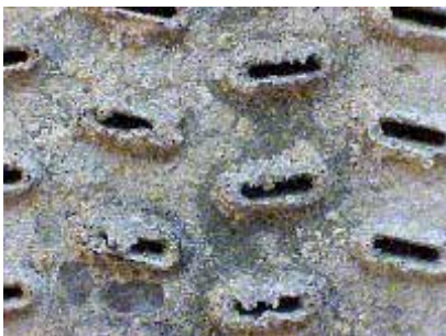
Resulting damage of poor coolant maintenance and/or poor water quality
